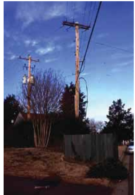
A wood fence and landscaping attempt to screen this voltage box from passerbys.
