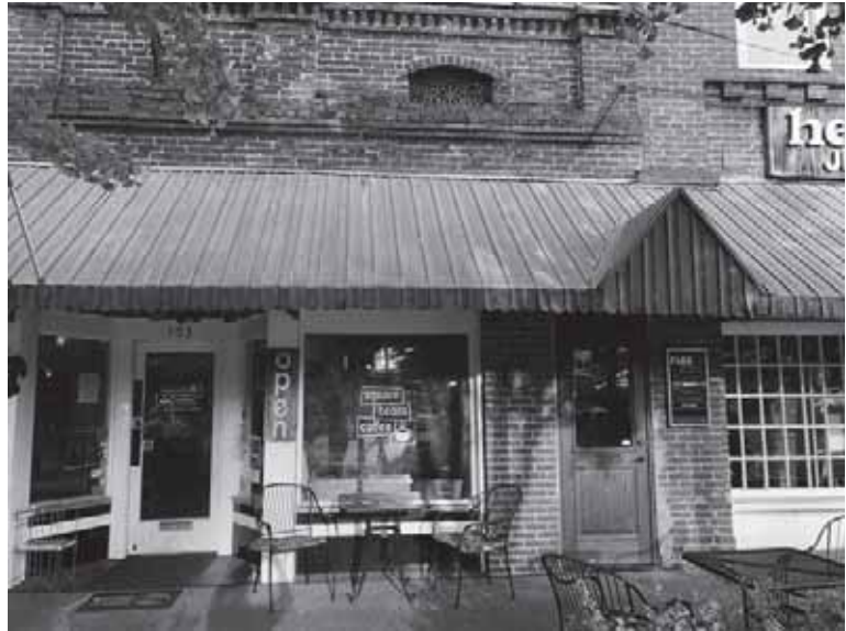
Widely available by the 1950s, aluminum awnings made with slats called "pans" typically arranged vertically were added to some storefronts. Aluminum "slat" awnings like these can be retained if original but should not be added where they do not currently exist.
