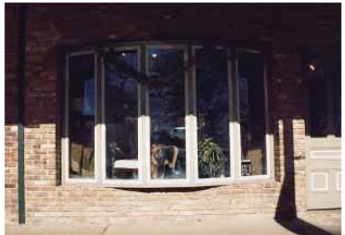
This retrofit display window is more residential in design and is not appropriate for a historic commercial building.
