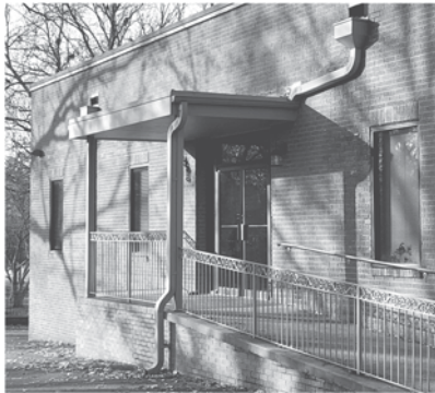
Metal canopies need to be properly maintained to make sure they don't rust.
