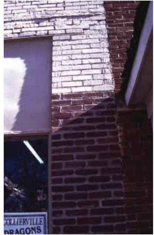
The re-painting of a brick building should be done carefully and thoroughly.
