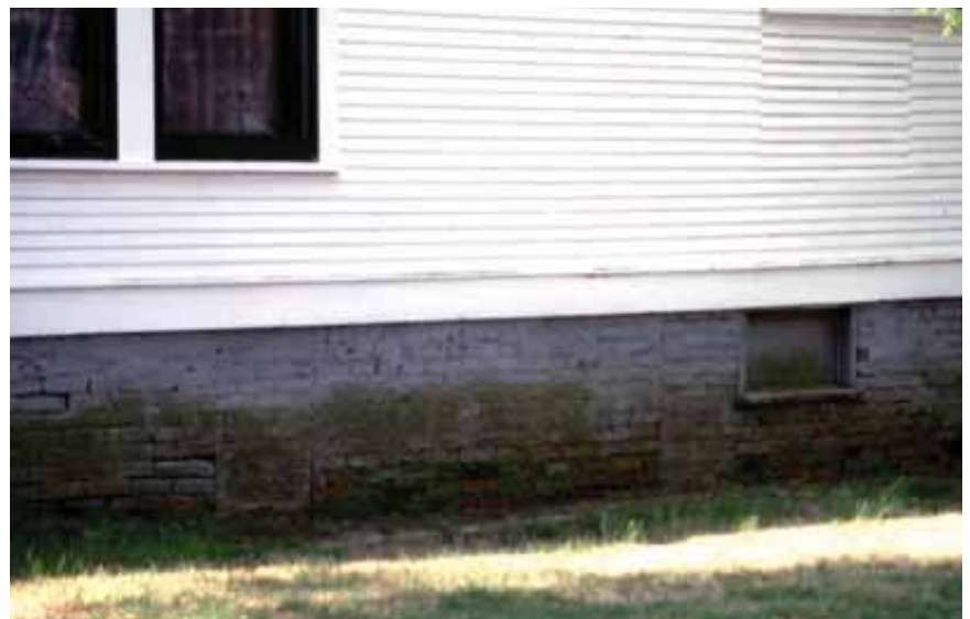
Brick is a common material used for foundations like this one found throughout the district.
