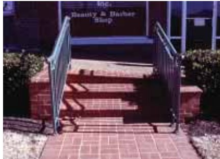
A stair leading to an ADA accessible ramp in the Town Square.
