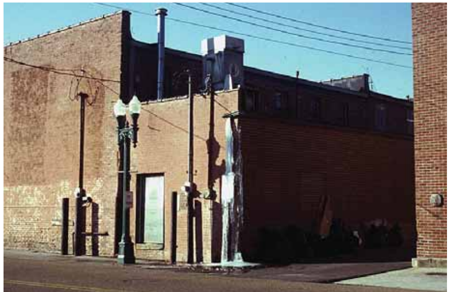
Maintenance of secondary elevations of a building is very important, especially when the elevation is in the public view.
