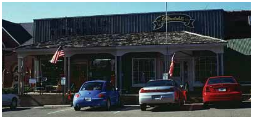
Artificial siding hides original materials on a building and is not compatible to surrounding structures.
