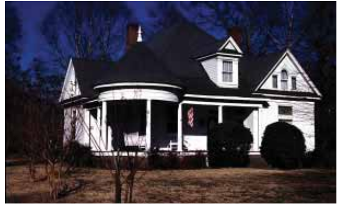
Asphalt shingles are not as appropriate for historic houses as is replacing with more historic materials.
