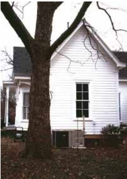
This air conditioning unit is located to the rear of the house, providing effective screening from the public eye.
