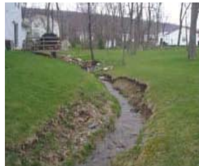
Poor stream buffer
