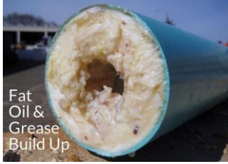
*FOG – Fat, oil and grease build-up
