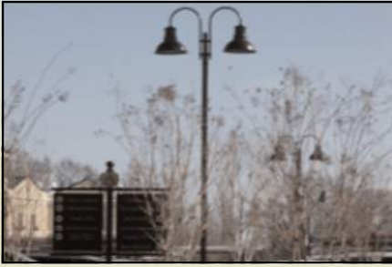
Fully shielded decorative light pole fixture
