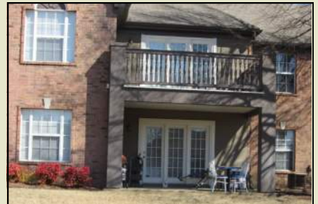
This ground level porch is not adequately screened
