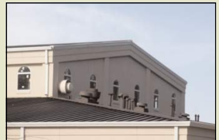
Exposed rooftop equipment is not permitted
