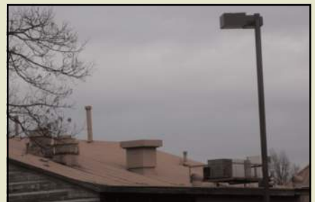
Unacceptable exposed rooftop equipment
